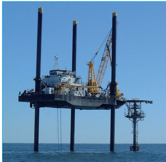
The liftboat Kayd is the mission-specific platform to be used during the New Jersey Shallow Shelf Expedition. Here it is seen being used to carry out repairs to a small platform in the Gulf of Mexico (photo D. Smith)
